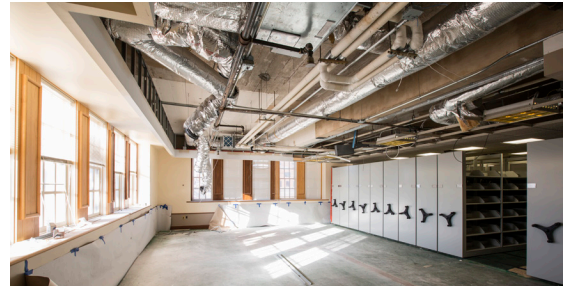
The compact shelving before renovations and the collection move. Simon Hurst Photography
